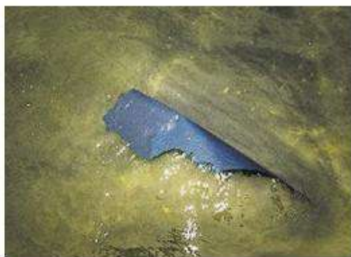
Recently applied blue paint appeared to be chipping.
